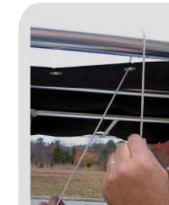
Bring the line over the pipe and down to the right side of line in "E".
